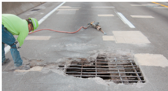
One of the many bridges that need repair on I-81
